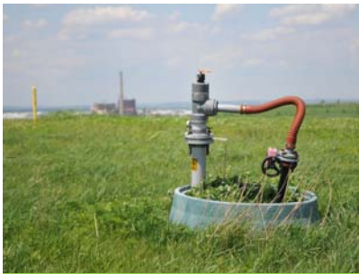
Landfill gas well
