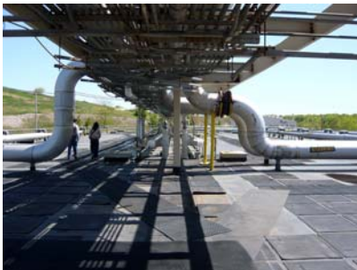
Leachate Treatment Plant
